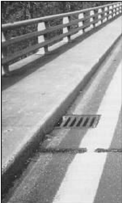
Figure 55 Example of pipes on a bridge
